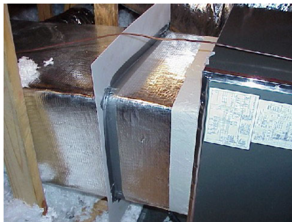
Figure 1. Supply Duct Blocked From Air Handler and Return Duct
